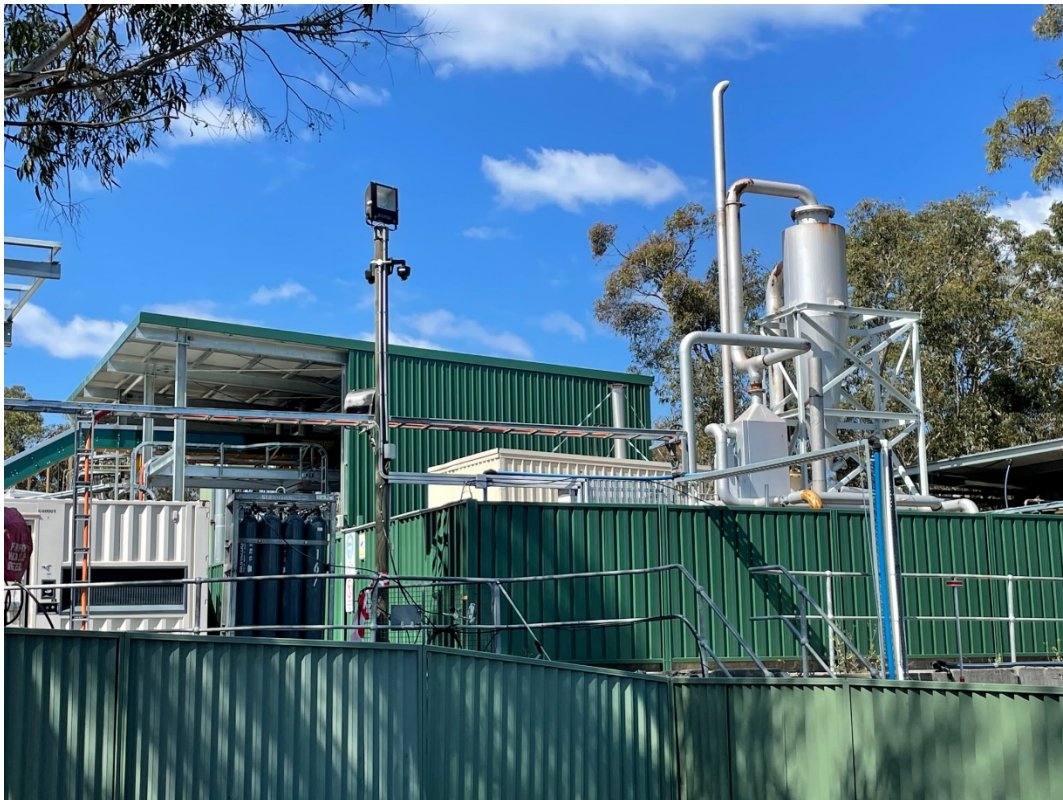
Image: The supercritical fluid boiler that heats the water for CS-1 at Licella's Cat-HTR ™ commercial demonstration facility in NSW, Australia.
