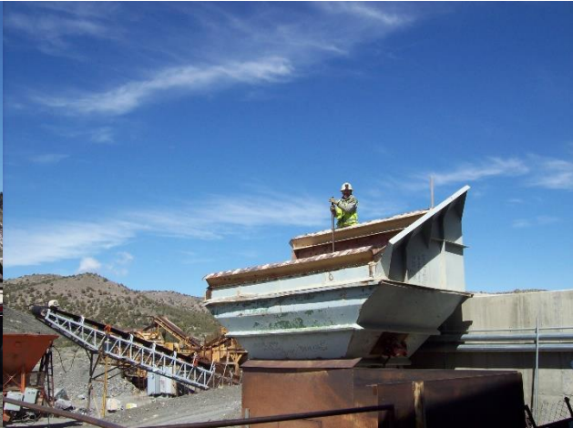
Receiving Hopper at Mill
